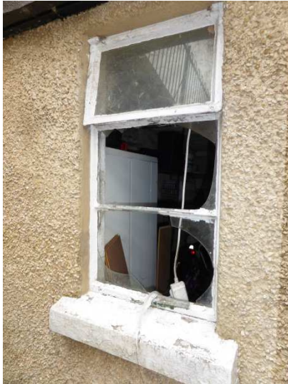
Damaged glass to windows will be replaced
